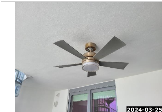
Rust Visible at Device
