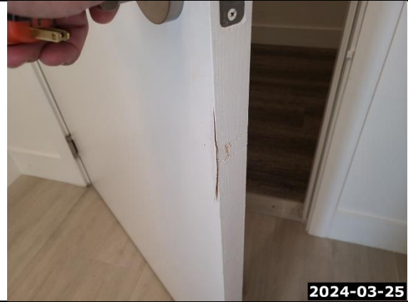
Damage at Front Door
