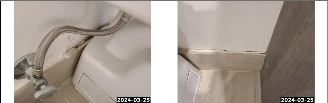
Grout / Caulk Damaged / Incomplete Behind Toilet Grout / Caulk Damaged / Incomplete Behind Toilet
