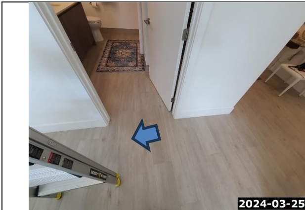
Tile Grout Damage at Main Walk / Hallway
