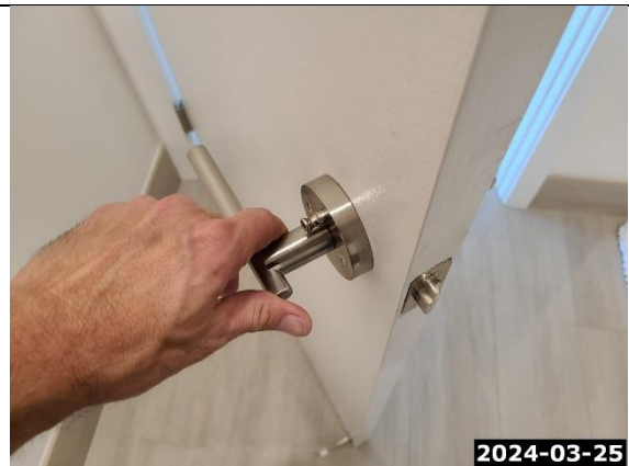
Loose Door Handle (Master Bathroom as Example)
