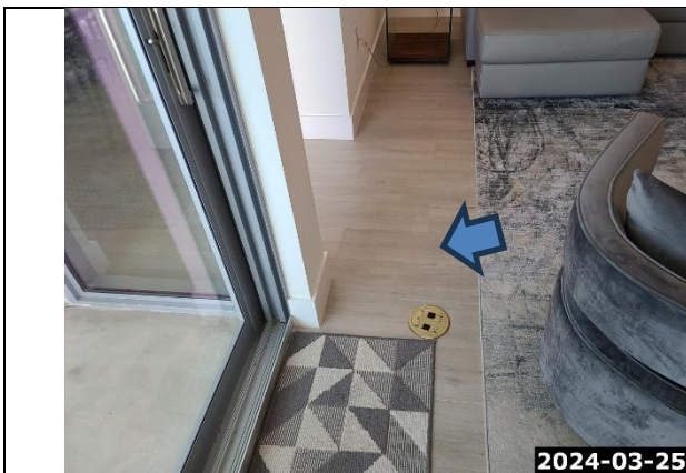
Tile Grout Damage near
