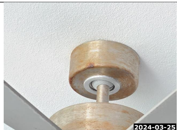
Rust Visible at Device
