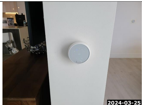
Wifi / Digital HVAC Thermostat
