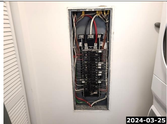
Interior Electric Panel (Cover Removed to View Wiring)
