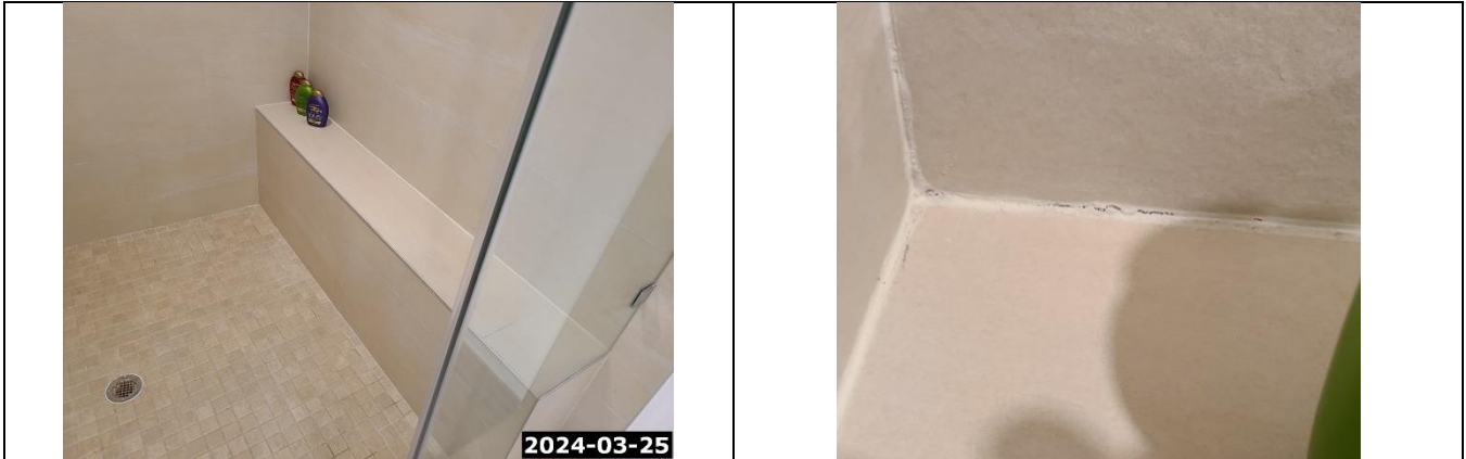
Bathroom #3 Caulk Cracking at Shower Seat Bathroom #3 Caulk Cracking at Shower Seat
