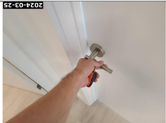
Northern Most Bedroom Door Handle Loose; Not Latching
