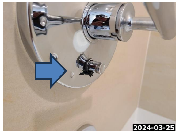
Material (Gasket?) Visible at Shower Diverter Button
