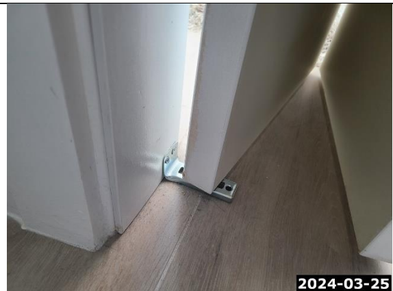
Anchor Attachment Appears to be in Incorrect Location
