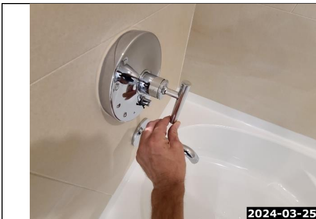
Bathroom #2 Shower Handle Loose
