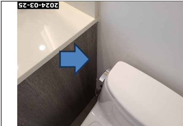
Caulking Incomplete at Cabinet
