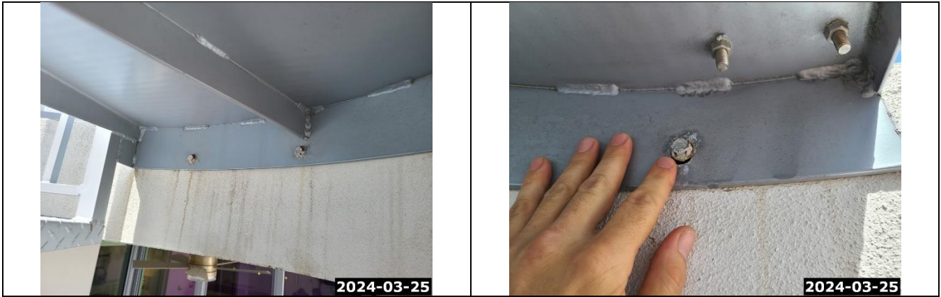
Balcony Staircase Seal Bolts to Prevent Corrosions Balcony Staircase Seal Bolts to Prevent Corrosions
