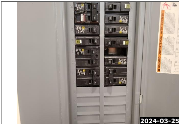
Cover Sitting On Breakers Instead of Around Breakers
