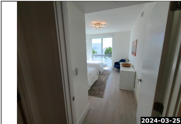
Northern Most Bedroom Door Handle Loose; Not Latching
