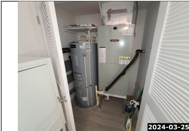
HVAC at Utility Closet
