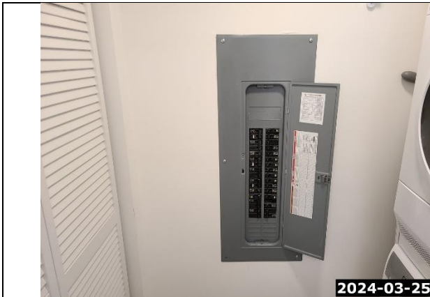
Interior Electric Panel (Cover In-Place)
