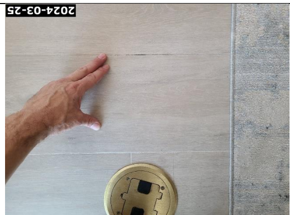
Tile Grout Damage near
