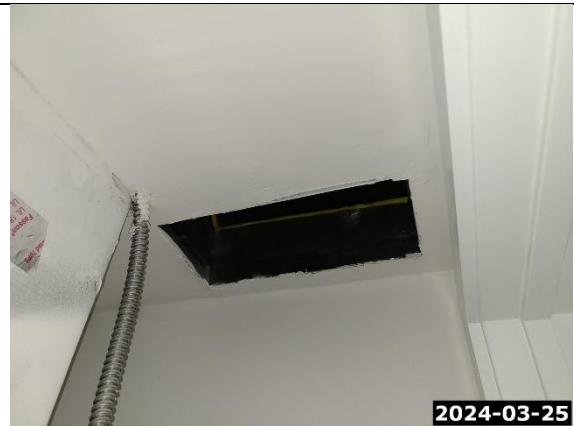
Opening in Ceiling in Utility Closet – Vent Register Required
