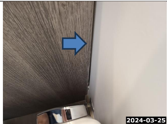
Caulking Incomplete at Cabinet
